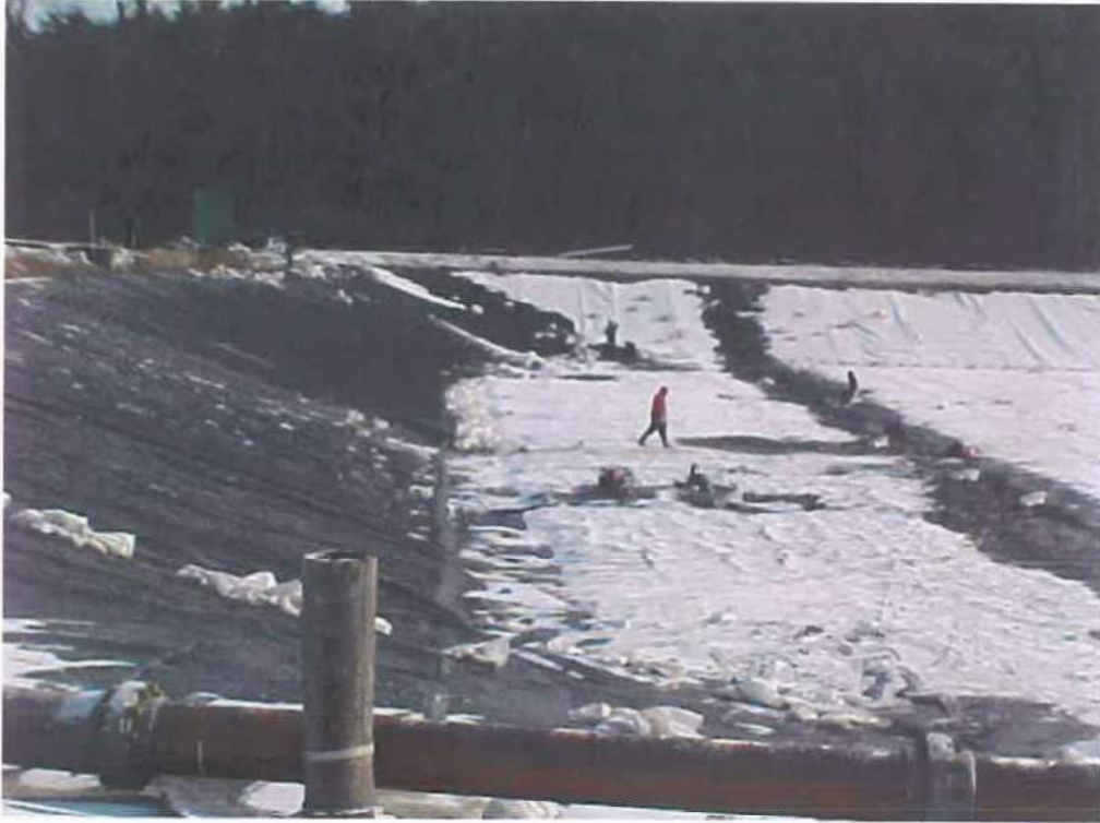
Photo 17 - Completed 60 Mil HDPE liner along the north slope viewing from west to east
