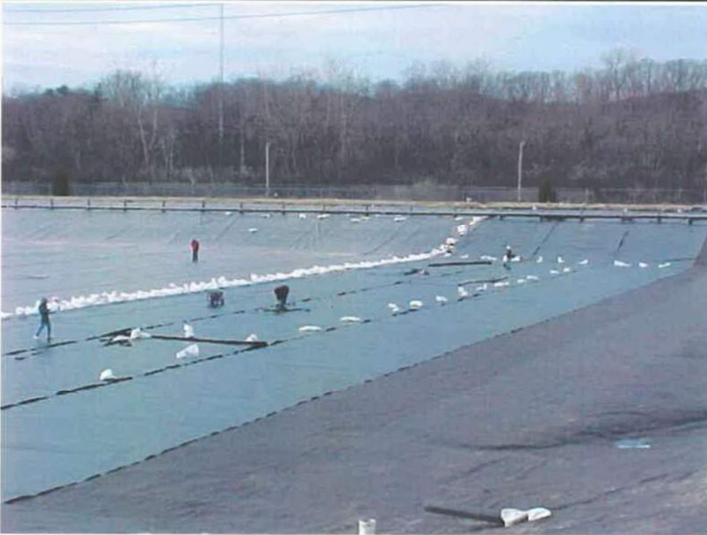
Photo 10 - Deployed 40 Mil HDPE liner viewing from the northeast corner looking back to the west
