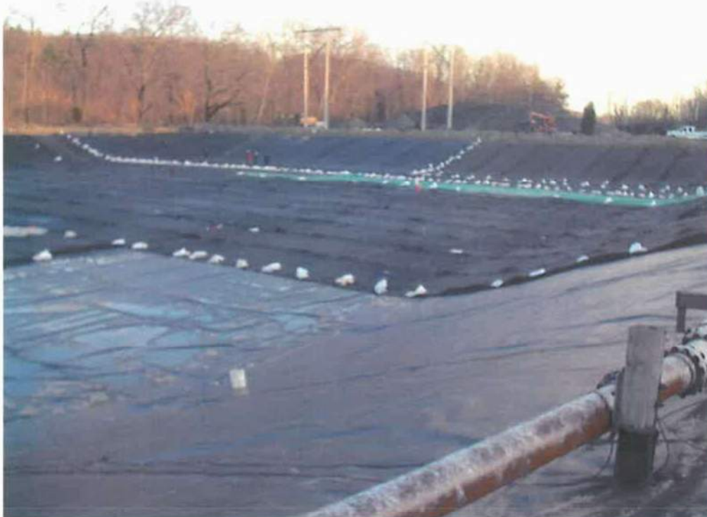
Photo 15 - Deployed geocomposite drainage layer viewing from the west back to the southeast
