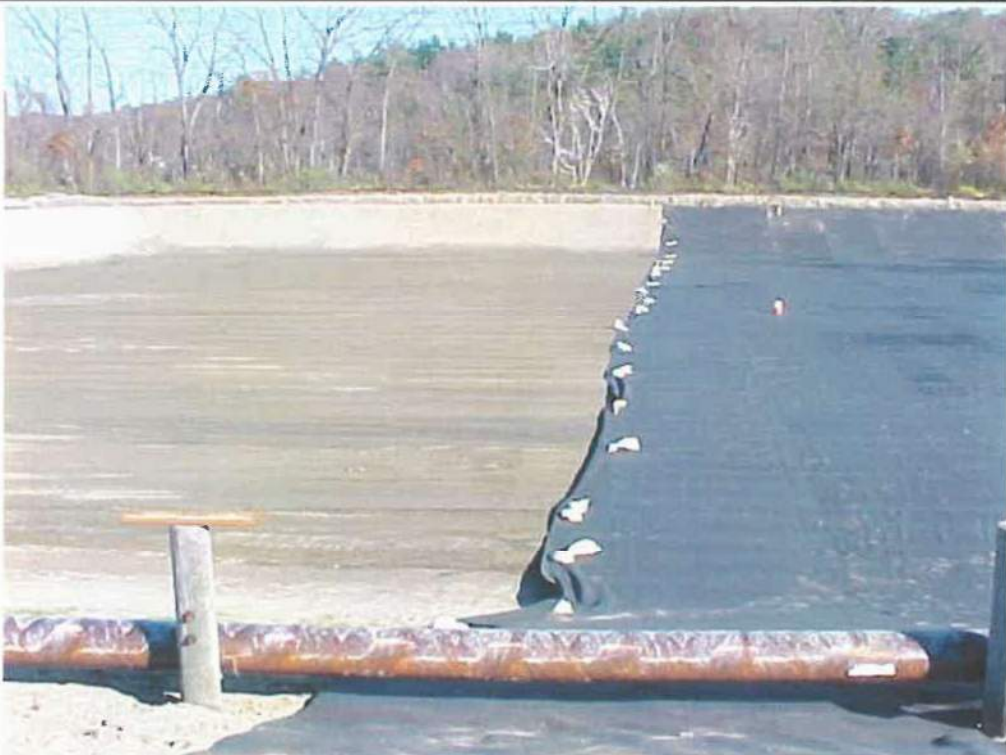
Photo 8 - Deployment of non-woven geotextile fabric, viewing from the west to the east
