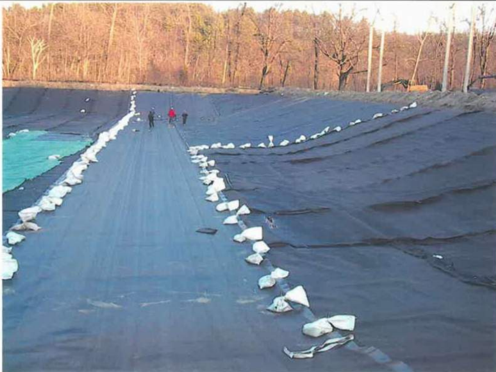
Photo 16 - Deployment of 60 Mil HDPE liner viewing the south slope from west to east
