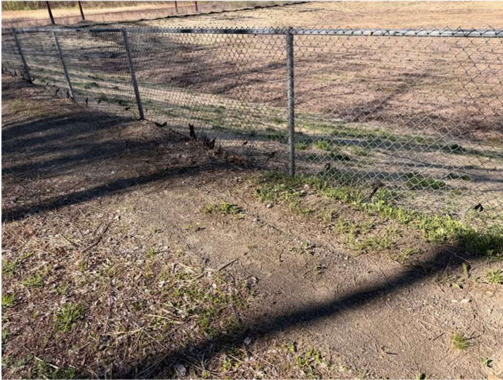
Photo 11 - Bare area on east embankment crest
