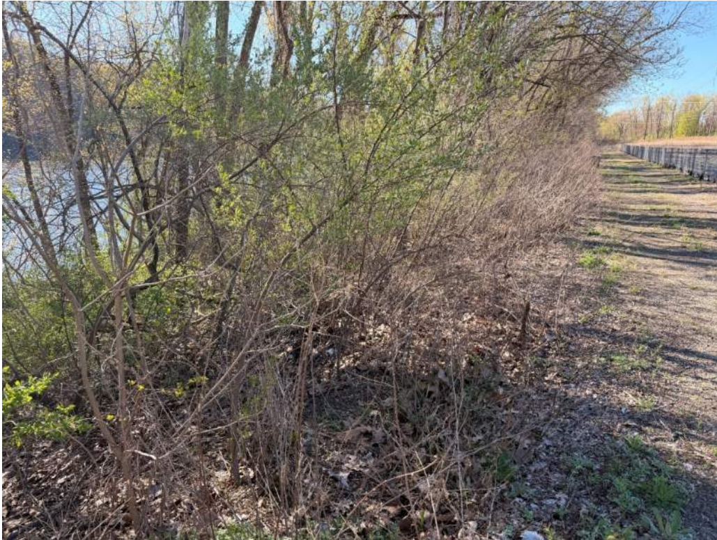
Photo 3 - East embankment exterior slope; note trees and brush
